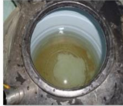
Drinking water Storage at Kakching Khunou Govt HS
